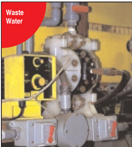
ARO 1/2" diaphragm pumps supply waste water treatment chemicals.
