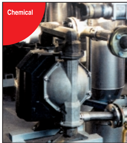
3" ARO diaphragm pump (located outdoors) transfer chemicals from train/truck tanks.
