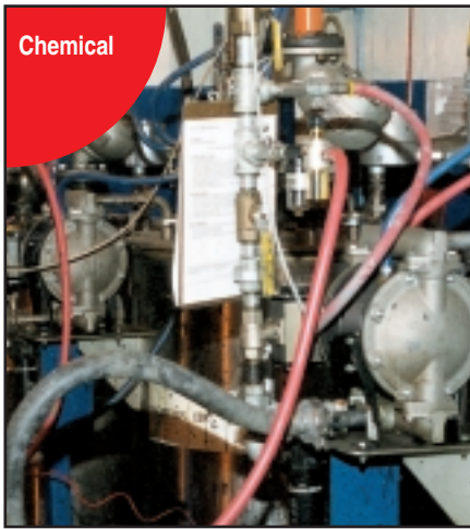
ARO 1" stainless steel diaphragm pumps transfer caustic material from 55-gallon drums into mixing tanks.
