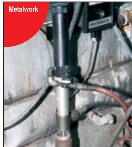
An ARO 2" piston pump supplies metalwork solvent.
