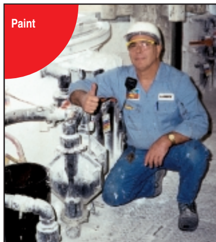
An ARO PD20A-X transfers paint formulation materials between tanks.
