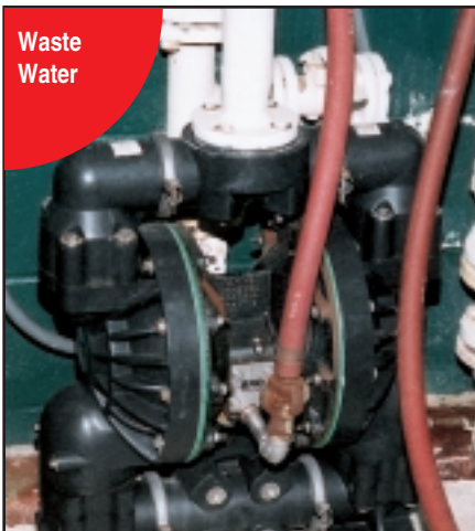
A 1-1/2' non-metallic ARO pump used in a waste water facility
